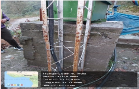
Visible rusting at Lattice poles of DTRs Village: Pakshep, Block: Mangan, North Sikkim
