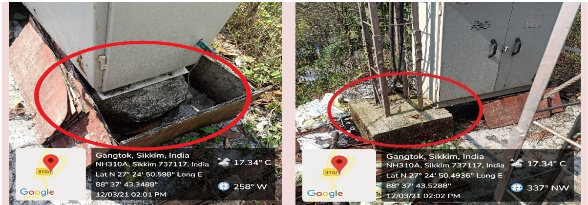
LTDB placed on stone and concrete base of lattice poles Village: Labi, Block: Kabi Tingda, North Sikkim
