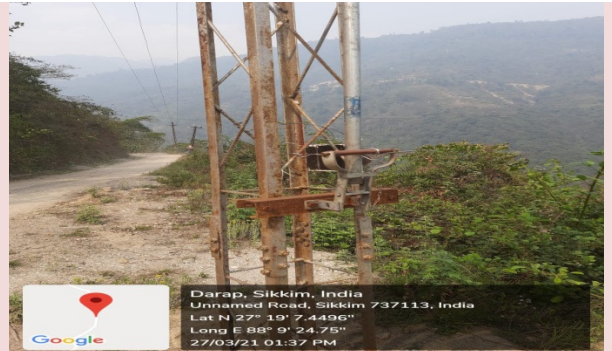
Visible rusting at Lattice poles Village: Nambu, Block: Gyalshing, West Sikkim
