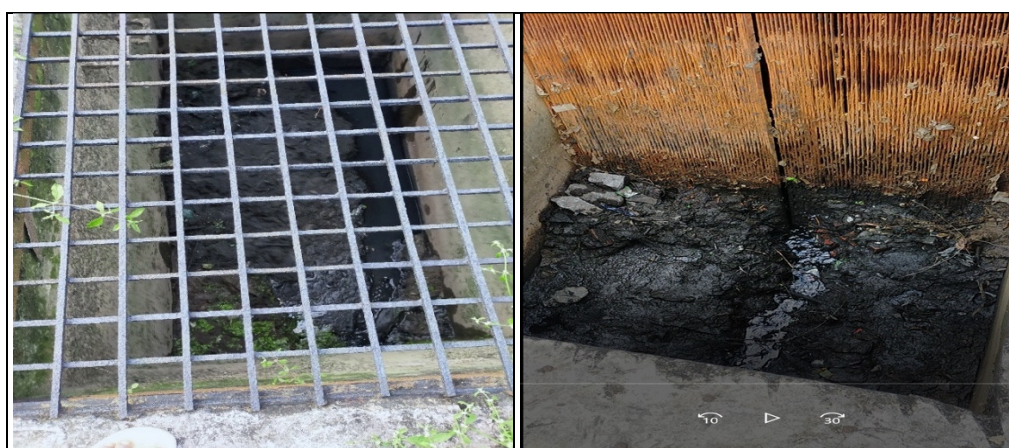
Picture 4.7: Chamber before STP-5 and the screen chamber of STP-5, filled with solid deposits
