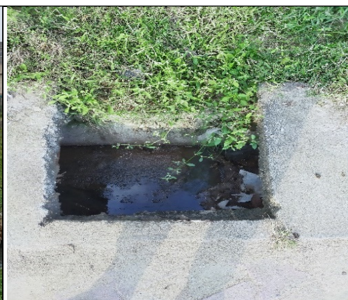
Picture 4.11: Stormwater drain filled with sewage
