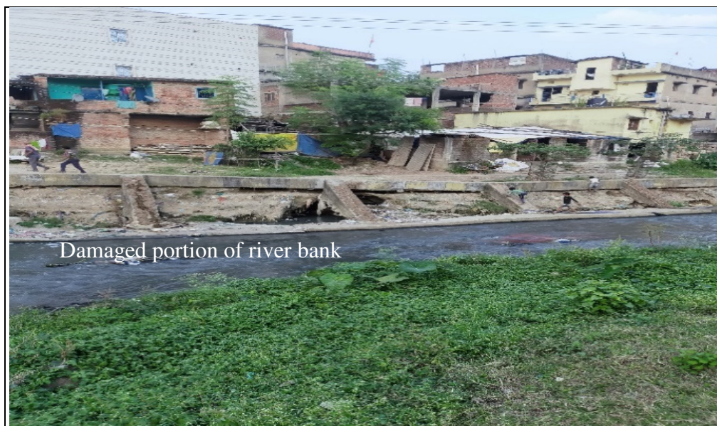
Picture 4.8: Damaged riverbank on the left side, between inlets 6B and 6C
