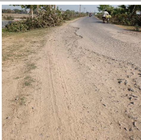
Fig. 2.14 Dilapidated condition of road
