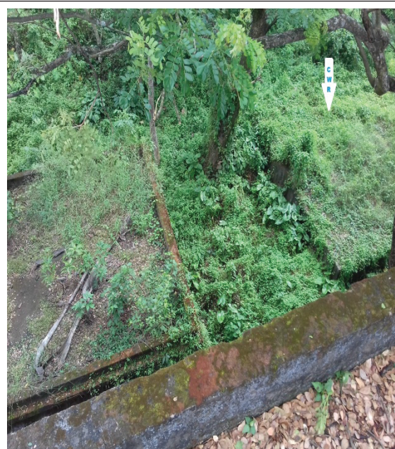
Fig. 2.13: Dilapidated condition of Clear Water Reservoir
