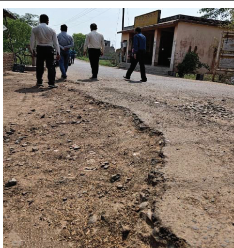
Fig. 2.17: Damage of edge
