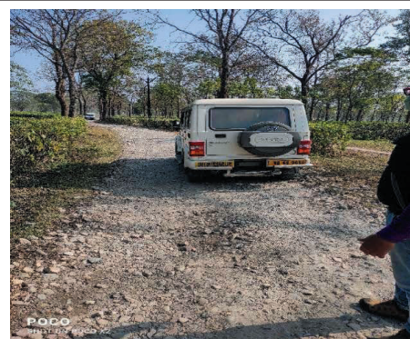
Fig.2.2: Worn out Bituminous surface at 14 km of road from Lalpur near Samuktala (20.12.2020)
