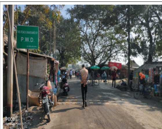
Fig.2.16: Encroachment of shoulder of Cross road by shops near Radhamadhav Mandir and Kaljani Housing complex under Alipurduar PW Division (20.12.2020)
