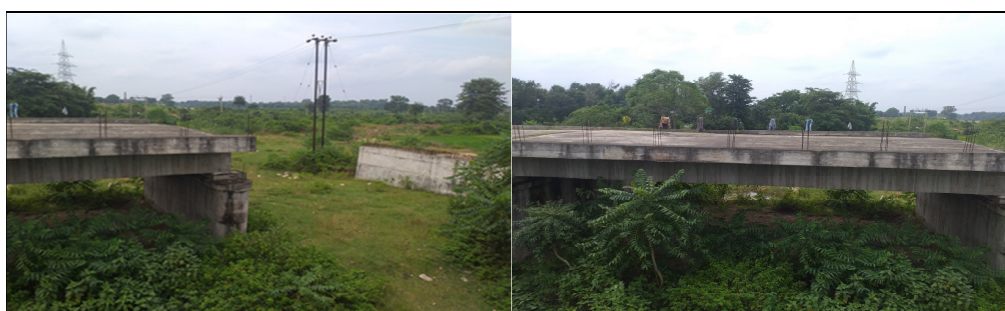
Photographs (taken on 18 September 2021) of incomplete bridge on Chouparan-Chatra Road over Baxa river
