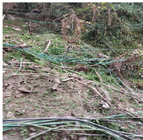
Water distribution pipes near Pani House, Gangtok
