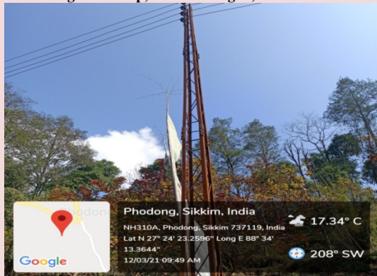
Unpainted LT pole Village: Phodong, Block: KabiTingda, North Sikkim
