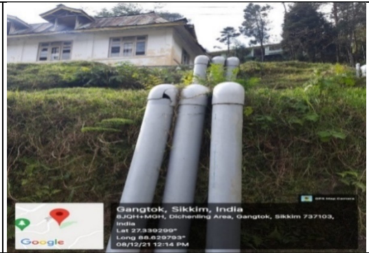
Image 4: Damaged PVC pipe at Enchey School where work was ongoing
