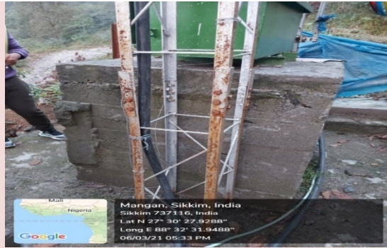
Visible rusting at Lattice poles of DTRs Village: Pakshep, Block: Mangan, North Sikkim
