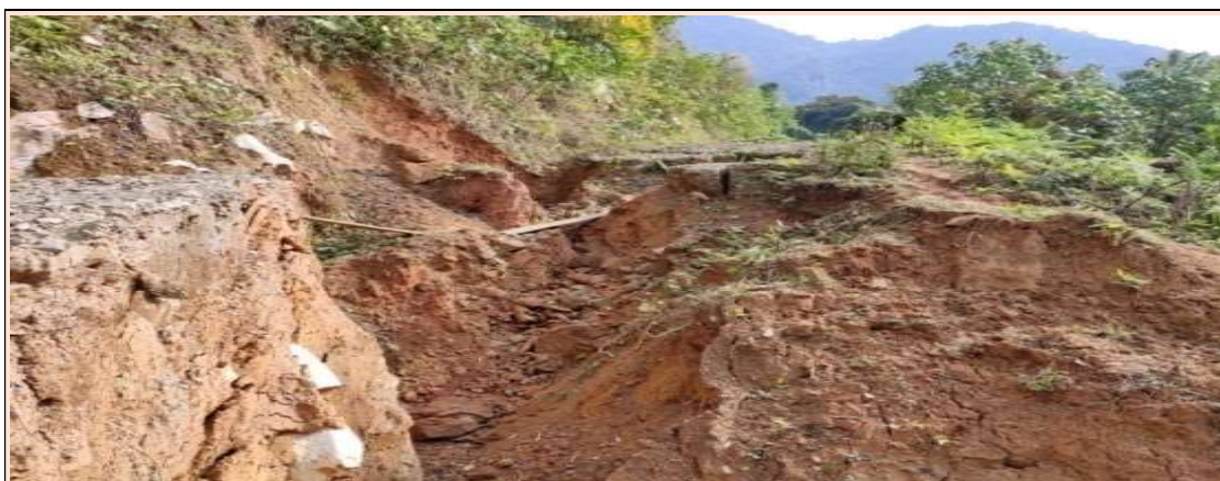
Chainage 4.200 Km: Road was not accessible beyond 4.20 km
