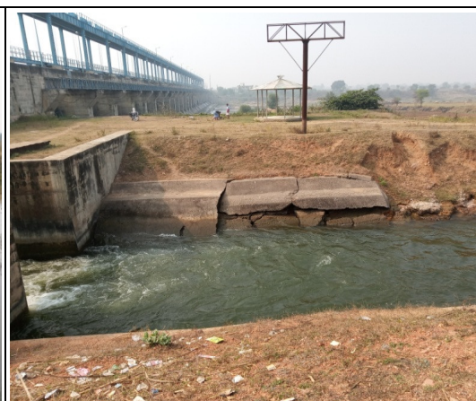
View of broken lining of Right Bank Canal (Beyond Mahuar River), near Samoha pickup weir. (Status: December 2019)
