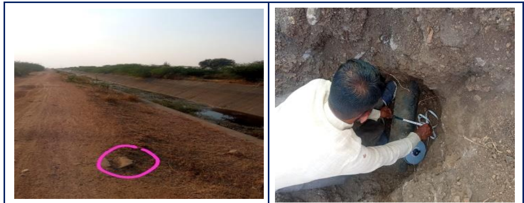
Exhibit 4.11: Incomplete pipeline work
