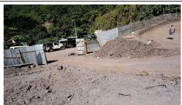
Dumping of topsoil along the roadside without providing any gullies/drainage channels at Mawlong area under DFO(T), Shillong
