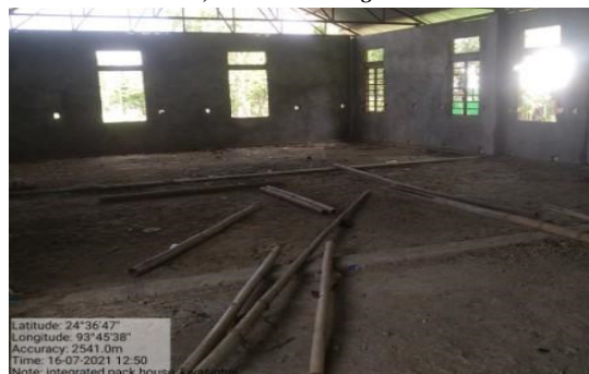
Incomplete Integrated Pack house of Integrated Rural Area Development Organisation (IRADO) at Kwasiphai, Bishnupur
