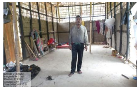
Pack house of L. Ichou Singh at Sansabi (Imphal East District) lying incomplete
