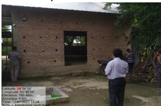
Pack house of L. Adenkumar at Khoijuman (Bishnupur District) lying incomplete
