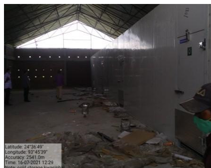
Incomplete cold storage unit at Kwasiphai
