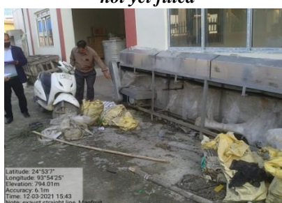
Straight line exhaust lying exposed
