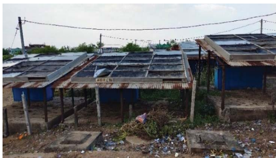
Fig. 34: Damaged Solar Panels at Nolia Nuagaon
