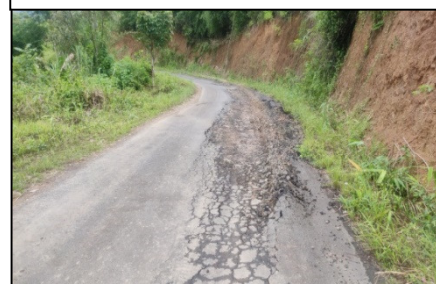
Photograph showing multiples potholes on the stretch of completed 9.5 Km
