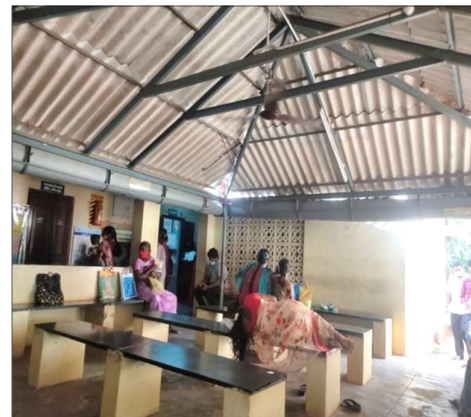
Exhibit 3.8: OP counter functioning under asbestos sheet at Urban PHC, Modakuruchi
