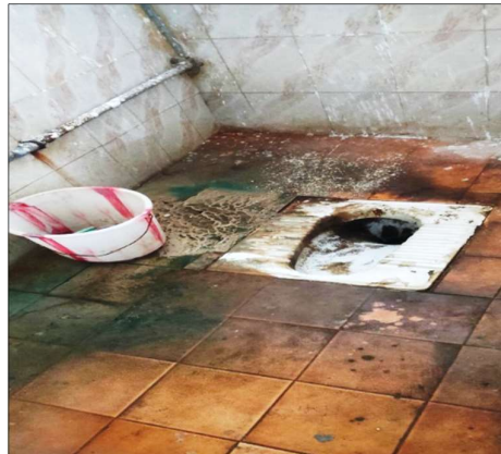
Exhibit 3.7: Unclean toilet at Urban PHC, Vettavalam
