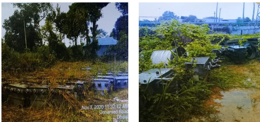
Transformers lying at open space, muddy surface, covered with bushes at Ambassa Store yard in Dhalai District
