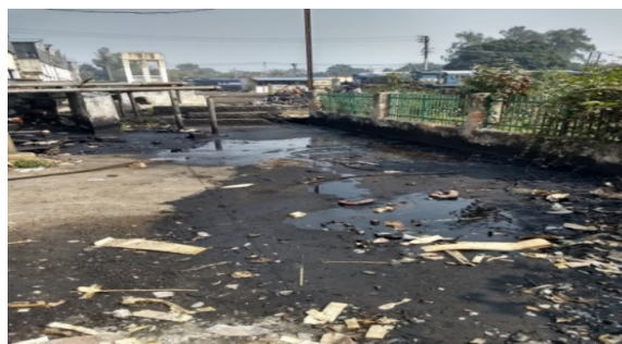
Hazardous waste lying in open space at Electric Loco Shed/Gonda of NER
