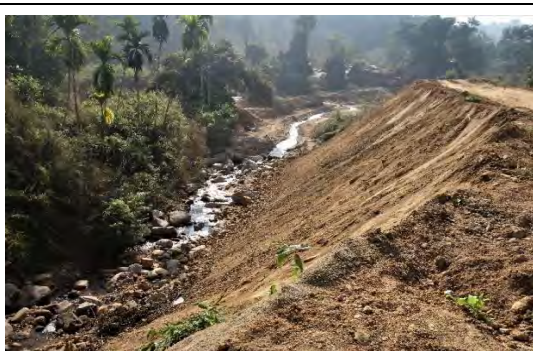
Dumping of topsoil along the bank of the stream at Mangapara area under DFO(T), Tura
