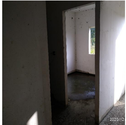
Water clogging in 1BHK flat
