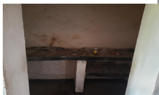
Damaged kitchen slab
