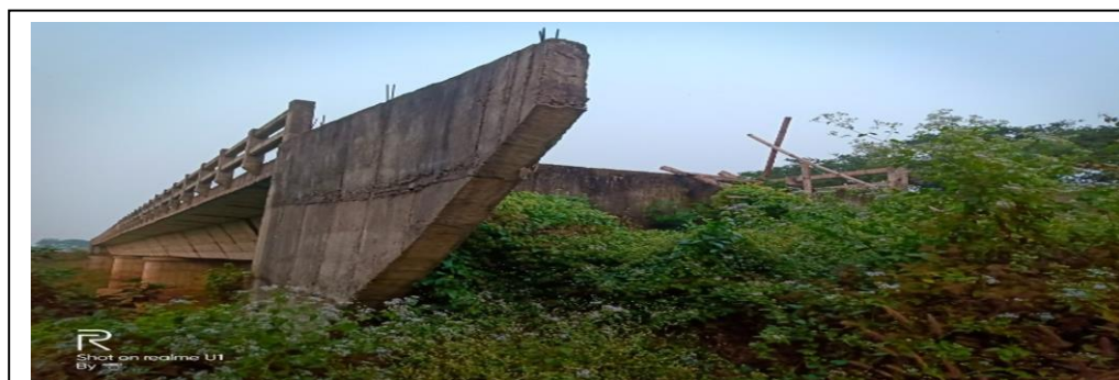
Non-construction of approach road to bridge over Sapua Nallah
