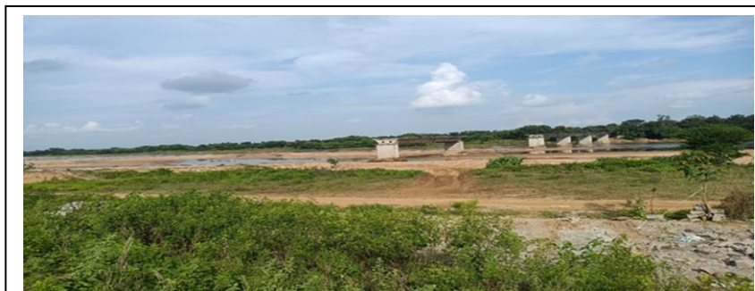
Incomplete bridge over river Lanth on Badipada PMGSY road
