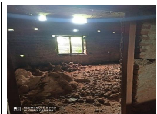
Incomplete building filled with ant hill in Jajpur
