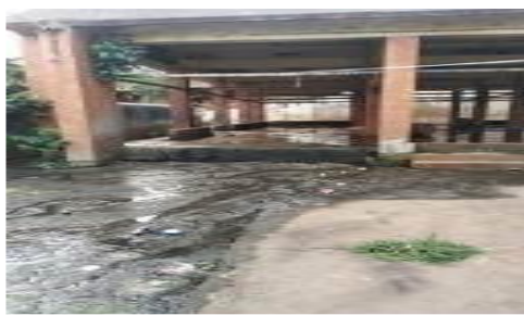
Photograph 40: Dilapidated slaughter house at Khannagar of CMC
