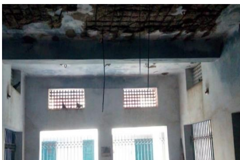
Roof of the day care centre at WWH, Balasore damaged
