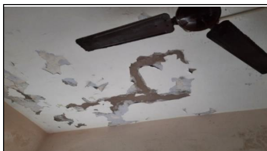
Nivedita WWH, Rourkela Damaged roof slab of a room
