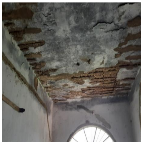
WWH, Balasore: Rooms of the first floor in damaged condition
