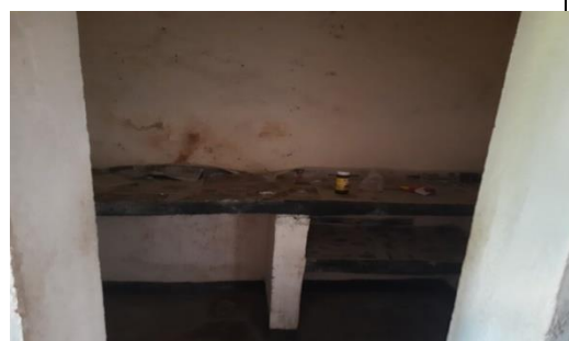
Damaged kitchen slab
