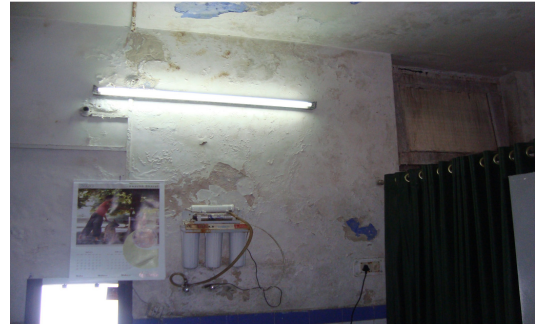
Photograph-17: Seepage in OPD (Ortho room) at DH Haridwar
