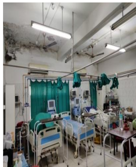
Pic 2.1.1: Bad condition of roof of HDU unit in Suri DH
