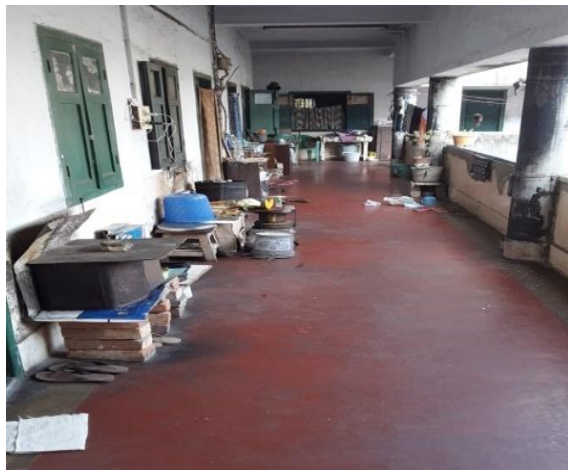
Pic 2.4.3: Boarders utilizing the common corridor for kitchen activities posing fire hazard in Gariahat WWH
