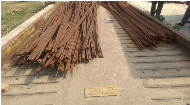
Pic 2.3.5: Construction materials being stacked on the unused Weigh Bridge platform at Tehatta KB Nadia
