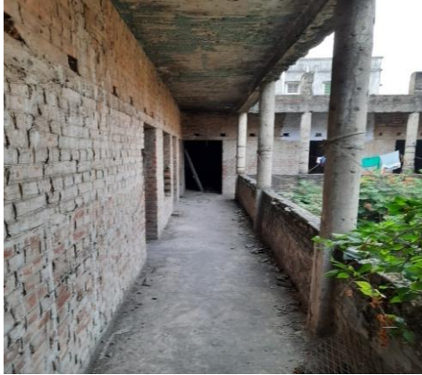
Pic 2.4.2: Incomplete first floor of WWH run by Shri Ram Krishna Ananda Ashram, Kolkata
