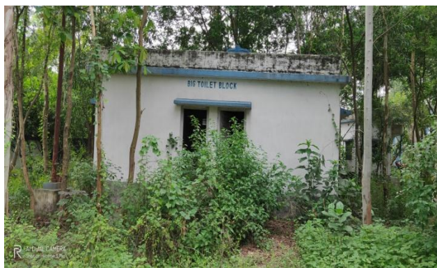
Pic 2.3.10: Toilets at Mayureshwar-I KB Birbhum becoming inaccessible by vegetation
