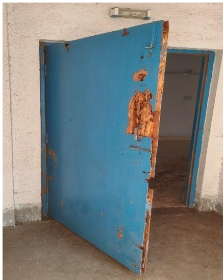
Pic 2.5.3: Badly affected door in PRMAS hostel, Talberia, Purulia
