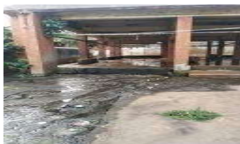
Photograph 40: Dilapidated slaughter house at Khannagar of CMC
