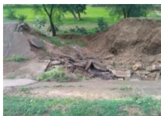
Breach in embankment near Phukujodi village
