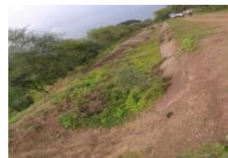
Sliding & silting of lining near Phukujodi village
