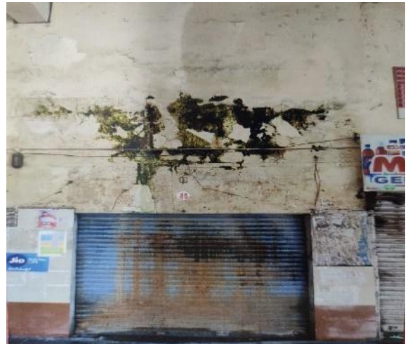
Picture No. 6.3.14: Water seepage at Madikeri bus station (May 2019).
