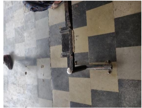
Picture No. 6.3.11: Malavalli bus station- Missing chair (May 2019).
