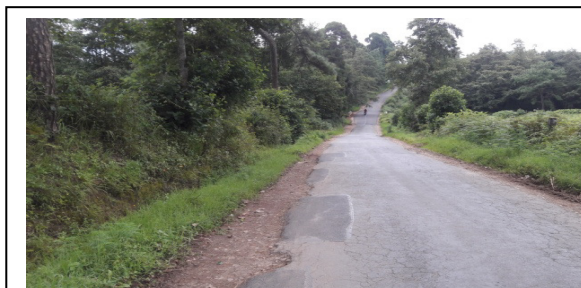
Picture showing the repair work undertaken (Nov – Dec 2017) at a cost of ₹1.70 lakh after the work 'Widening i/c MBT of existing pavement of Shillong Peak Road - under RIDF-XX' which was completed in December 2016. Date of joint physical verification: 07.08.2018
