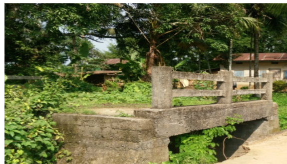
The work 'box cell culvert' against the main work 'Improvement i/c MBT of a road from Gimigre Old Model to Bollochiring (0.00-2.00km) under RIDF-XX' constructed at a cost of ₹ 13.76 lakh remained unutilised as the approach road could not be constructed due to land dispute. Date of JPV: 05/06/2018
