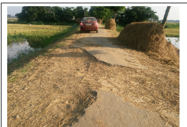
Picture showing broken road in the work 'Improvement i/c MBT of a road from AMPT road to Haribanga village via Bholarbita (0.300 Km) under RIDF-XX' which was completed during February 2017. Date of joint physical verification: 05.06.2018
