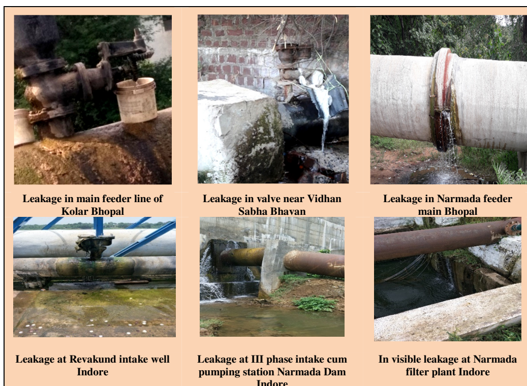
Photographs showing the leakages in main lines of MCs water supply
