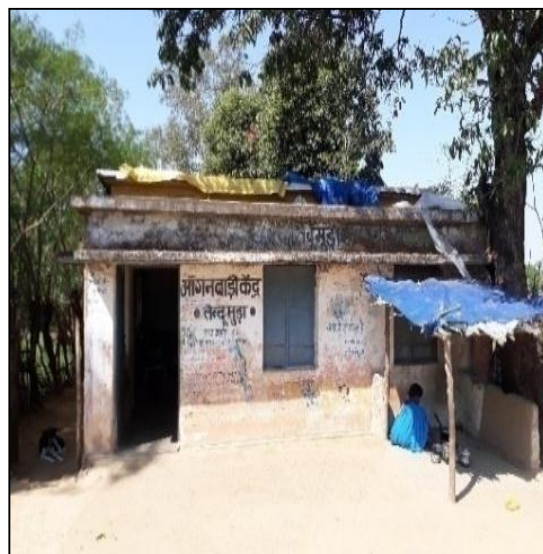
Photo 2.3.12.2 (b) - AWC Tendumunda (Gourella) dilapidated building (from inside) not being used and food was being cooked outside in open in temporary shelter
