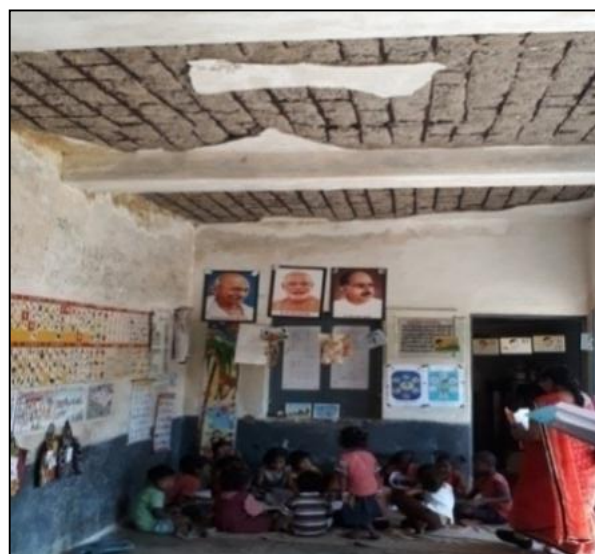
Photo 2.3.12.2 (a) - AWC Kolanpara (Gourella) operating in dilapidated building which poses safety hazard for children.
