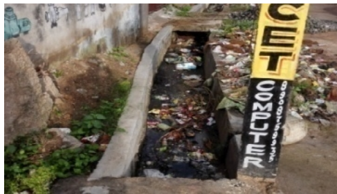
View of a choked drain
