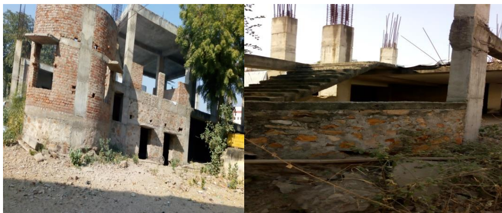
Incomplete building of auditorium at JLN Medical College, Ajmer
