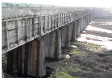
View of seepage from Karam aqueduct (Phase-II) (Status as on June 2017)
