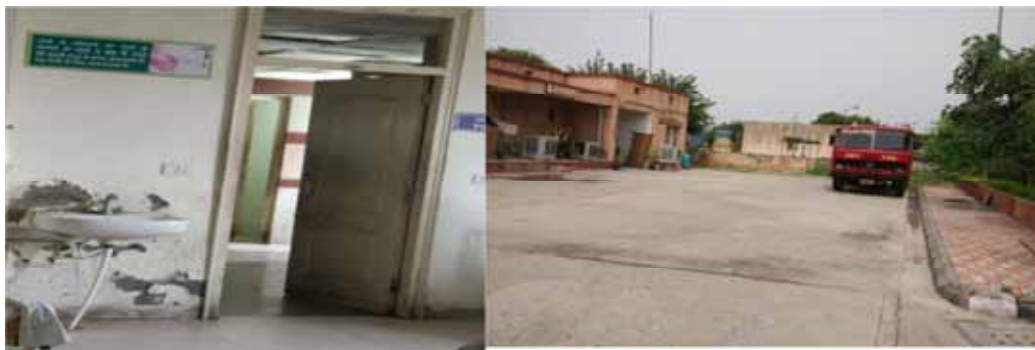
Seepage in the wall
