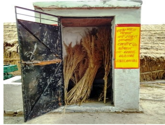
Plate 5.2: Non-functional toilet GP-Kirachan, Block Rajepur, Farrukhabad, Uttar Pradesh
