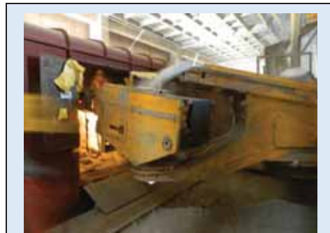
Mechanised loading of cement being done in a wagon in South East Central Railway
