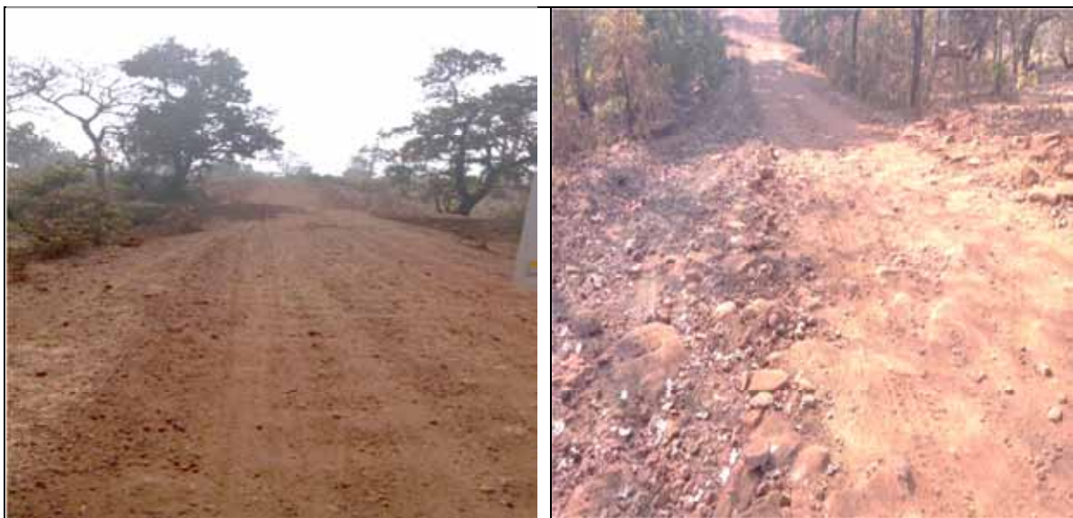
A view of incomplete work at km chainage 1,200 and 2,100 of Anarad to Nihaldevi road as on January 2017 due to delay in proposal for acquisition of forest land
