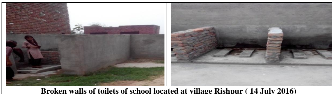
Broken walls of toilets of school located at village Rishpur ( 14 July 2016)
