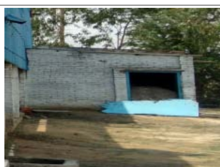
Hazardous waste storage without doors near Chak Ganjaria at Lucknow
