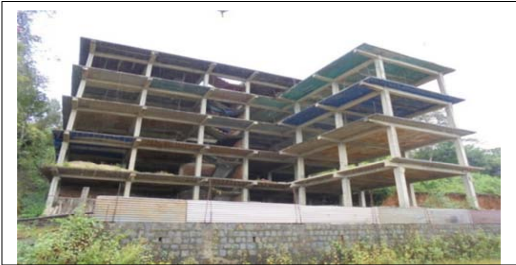
Photograph of Under construction building at New Secretariat claimed as budget accommodation
