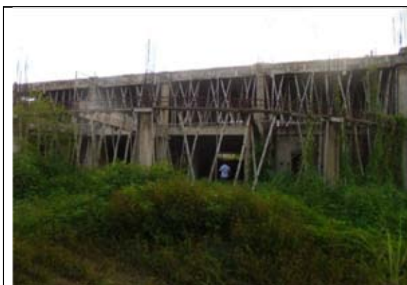
Photograph of abandoned construction of the Mega Destination Dimapur
