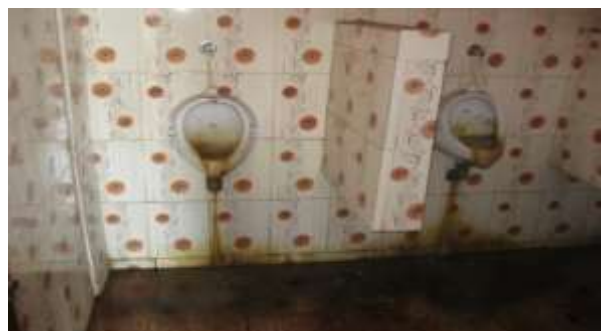
Water blocked closets in Municipal Complex toilet
