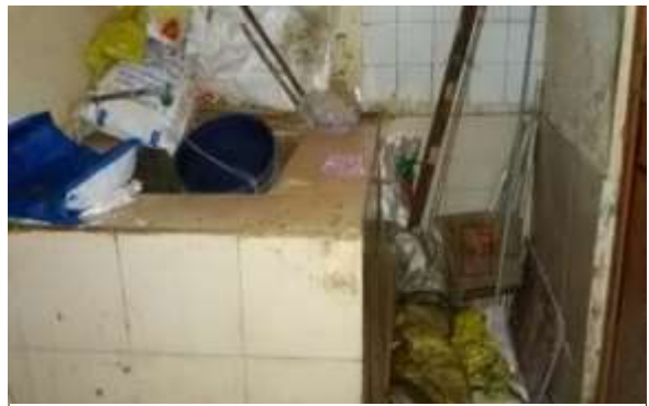
Waste dumped inside ladies toilet
