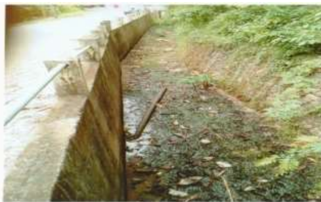
Septage dumped inside the canal at Elavakkad, Thrikkakara
