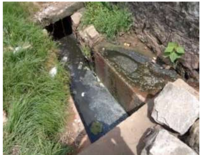
Blocked drain at Alamcode Fish Market in Attingal
