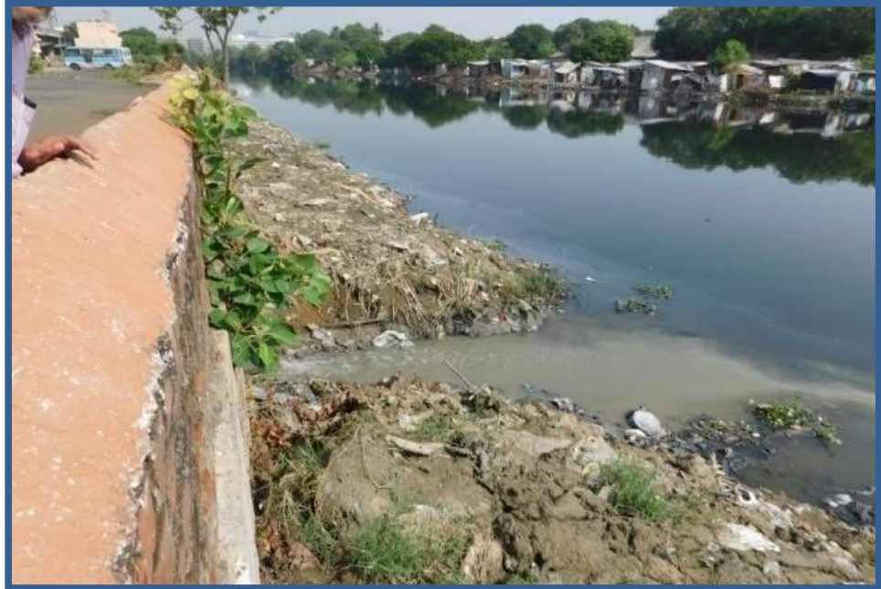
Encroachment and sewage outfall (Pallavan Nagar)
