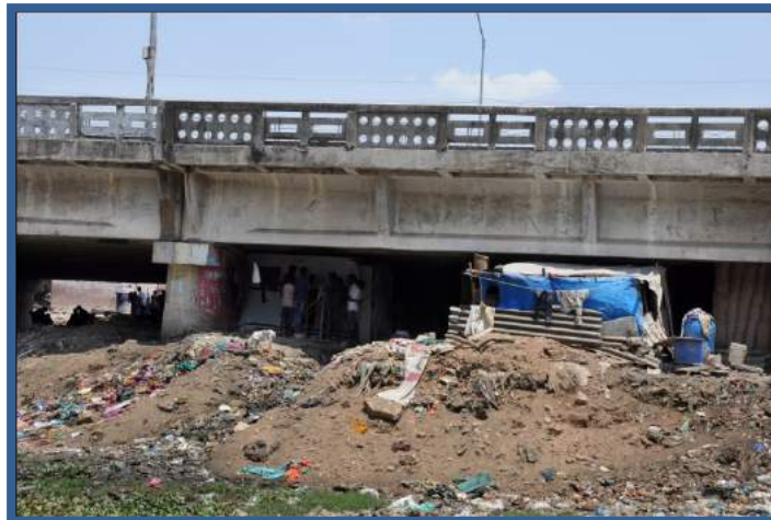
Exhibit 4.2: Encroachments in Maraimalai Adigalar bridge (with blocked vents)
