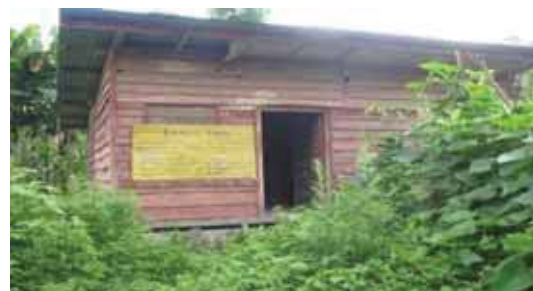
Picture-17: Poor condition of Labour Room of Maram Khullen PHSC, Senapati District Manipur
