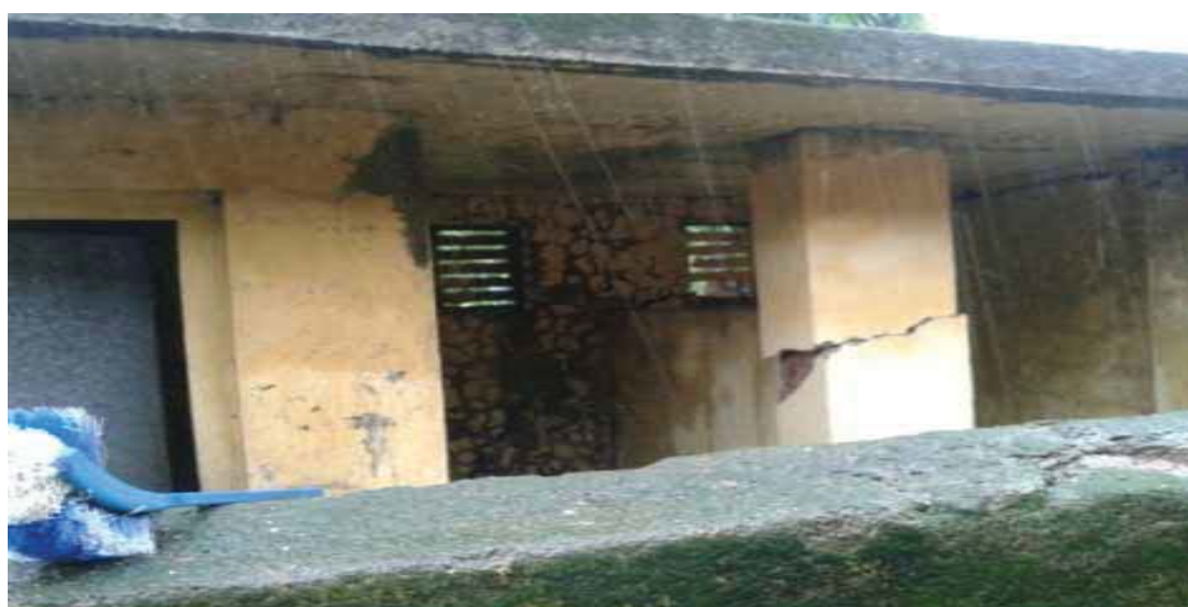
Picture-6: Toilet blocks of Upper Primary School, Varoli Talat, Valsad district, Gujarat, in damaged condition,
