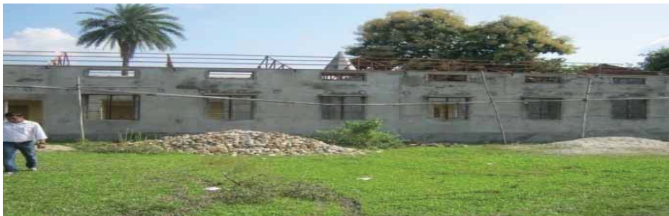
Picture-10 : Sankar Dev Mission high School, Udalguri, Assam – Building incomplete even after lapse of nine months from due date of completion
