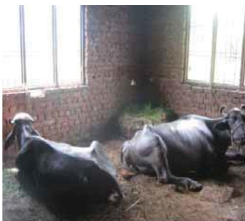
Picture-1: KGBV building (under Construction) Doongi, Rajouri, J&K being used by locals as cattle shed
