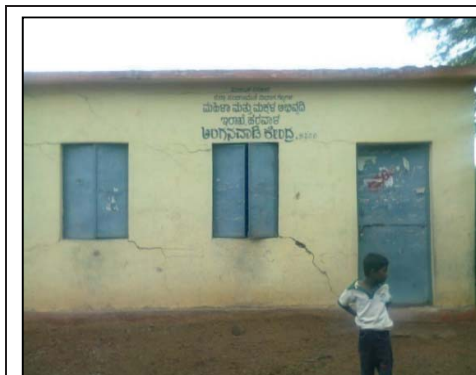
Poor quality construction of Anganwadi in Haravali village, Kalaburagi district (27.08.2014)
