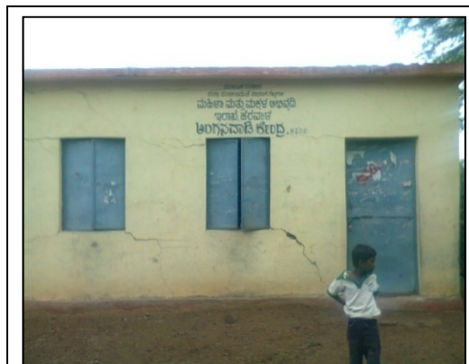
Poor quality construction of Anganwadi in Haraval village, Kalaburagi district (27.08.2014)
