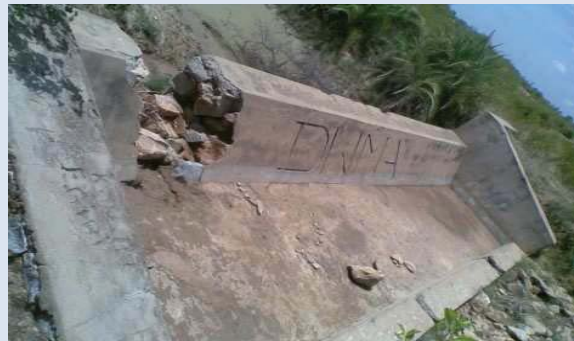
Name of the project: Chalkurthanda Name of the district: Anantapur Non-repaired check dam with toe wall and apron
