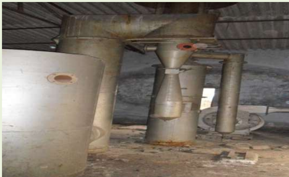
Incinerator lying idle in the premises of DH- Korba
