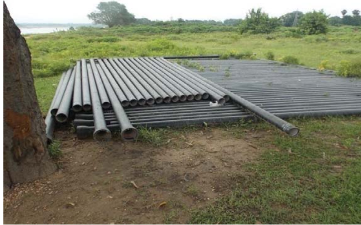
Figure :Kulti municipality pipes stacked without security
