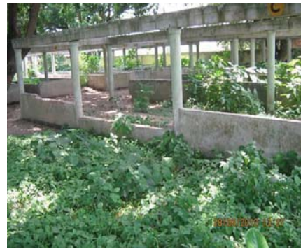
Dilapidated Vermicompost plant of model facility
