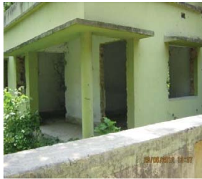
Dilapidated building of model facility
