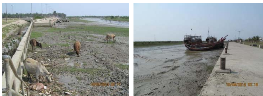
Heavily silted Minor Fishing Harbour at Harwood Point, Kakdwip
