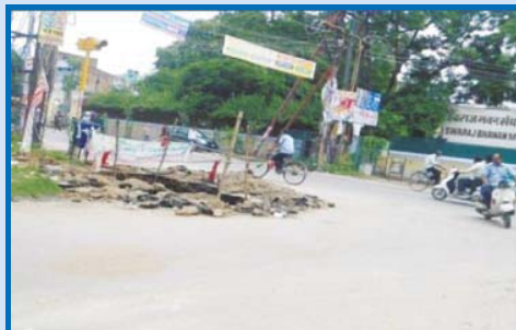
Damaged road-Anand Bhavan road, 01.07.2013.
