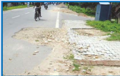
Damaged road-DPS-Omaxe city to Mirzapur road, 01.07.2013.
