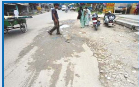
Damaged road-Rewa road, Dandi market, 01.07.2013.
