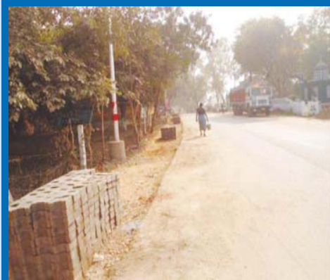
Railway Naini feeder road- interlocking work not completed as on 24.1.2013.
